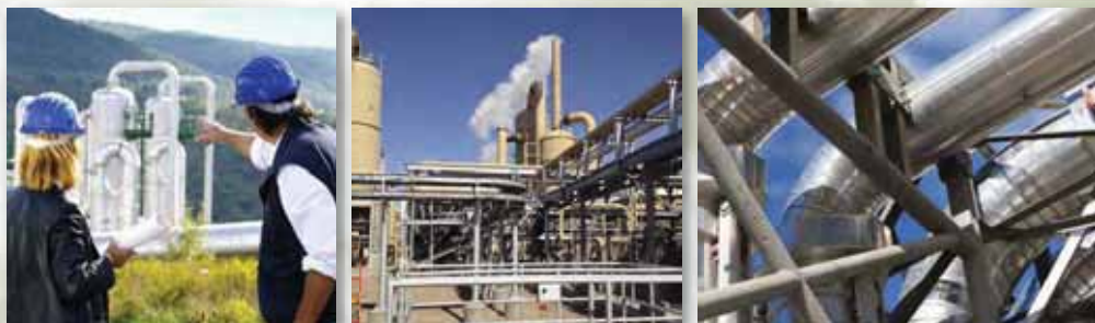
Hudson Ranch – the first new geothermal plant in the Salton Sea area in more than 20 years
