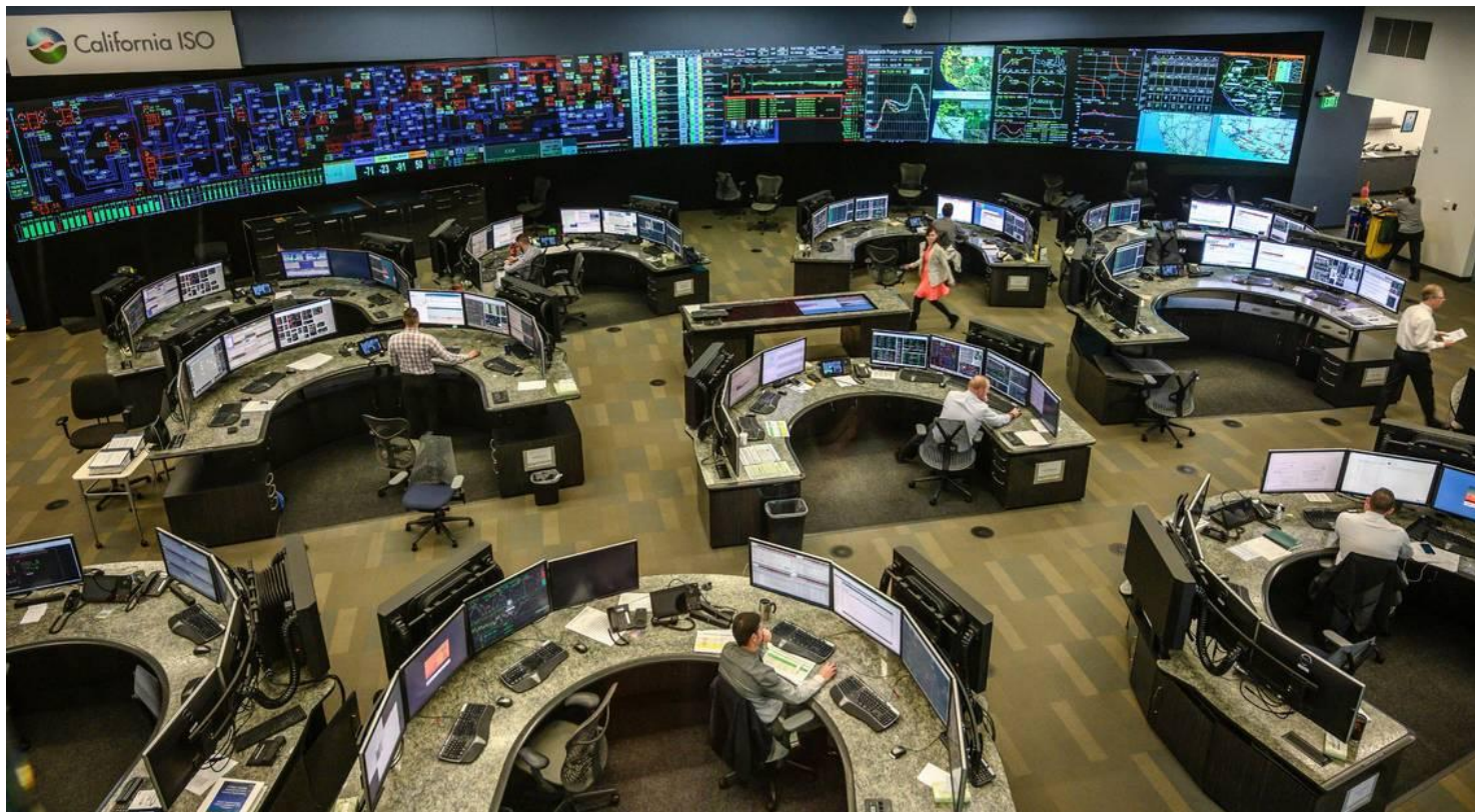
A view of the control room from an overlook room shows the power grid in 2018 at the California Independent System Operator in Folsom.
