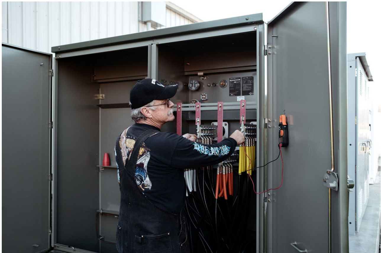
Randy Cox, the Blue Lake Rancheria tribe's electric system director, tests the microgrid transformers.
