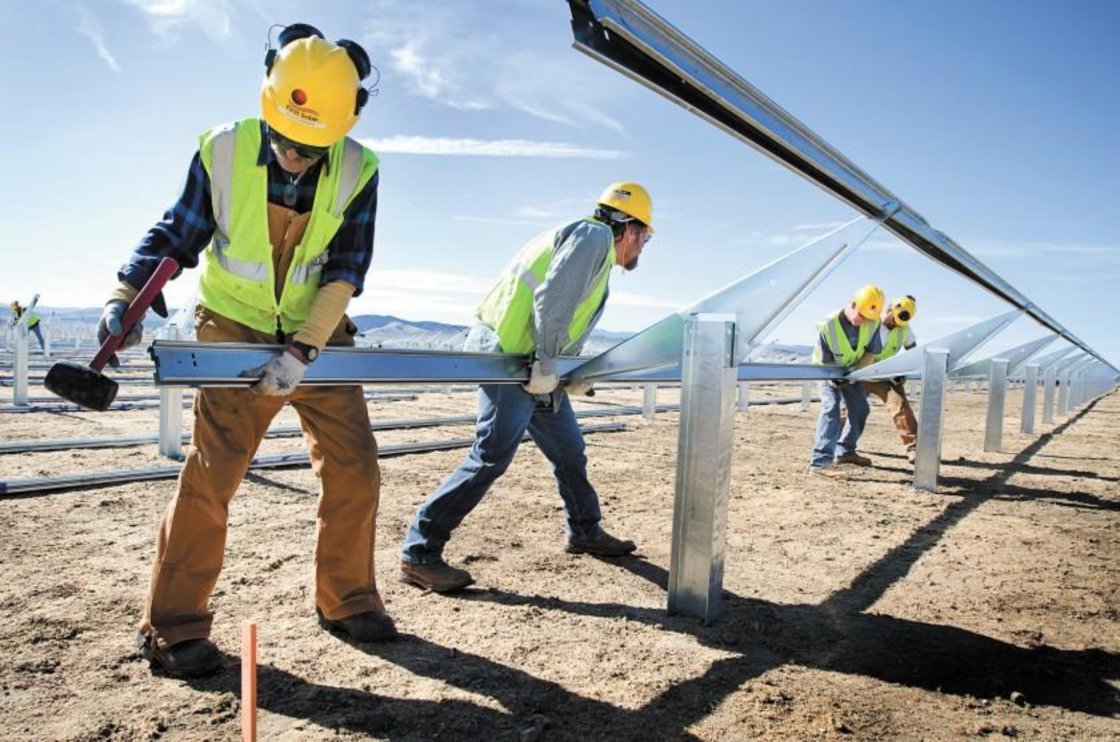
A crew installs rails to support some of the 9 million panels at the Topaz solar farm near San Luis Obispo. (Joe Johnston / San Luis Obispo Tribune)
