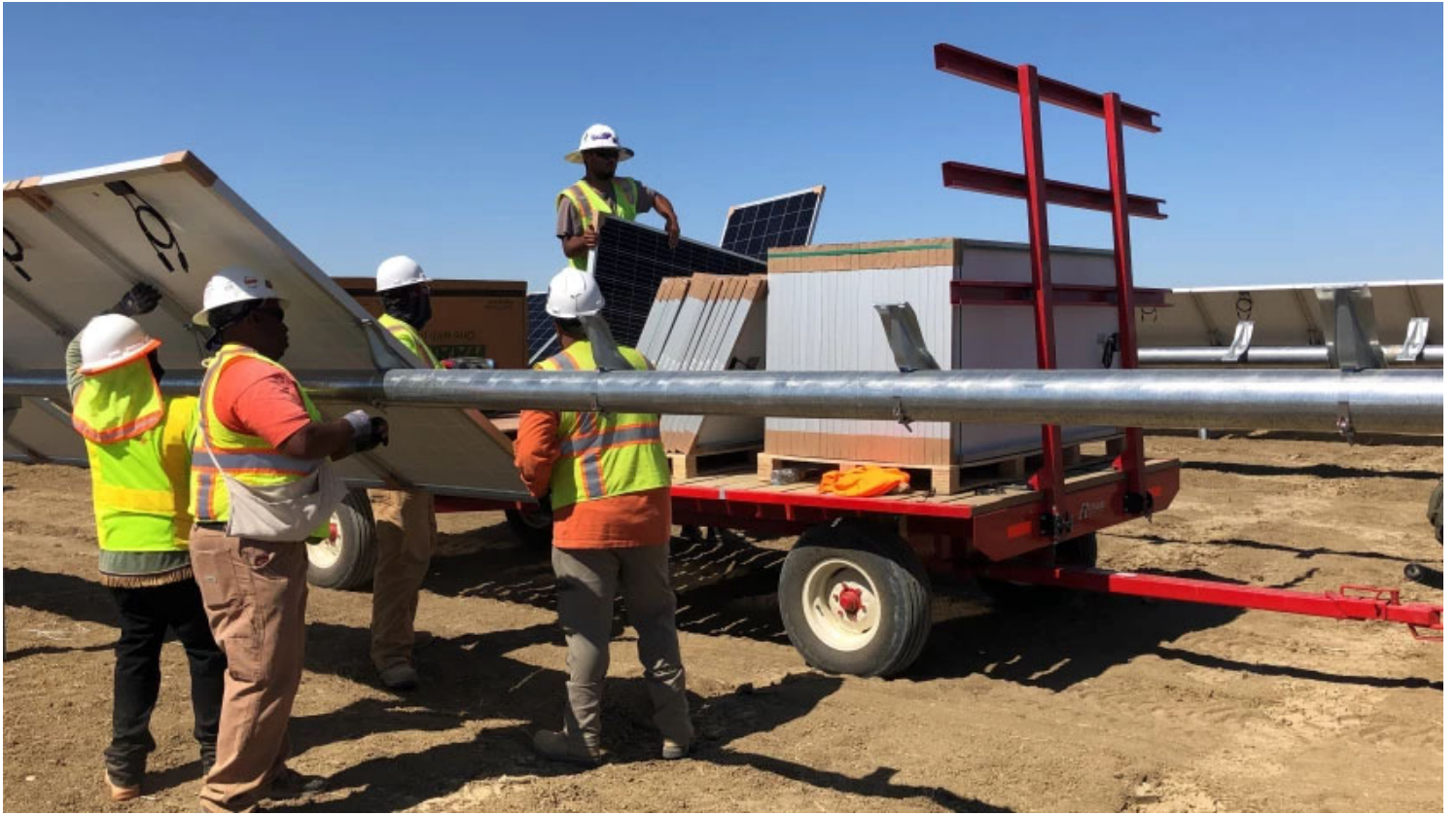
Construction workers at Westlands Solar Park project unload solar panels from a tractor, place them on steel racks and screw them into place. (Sammy Roth / Los Angeles Times)
