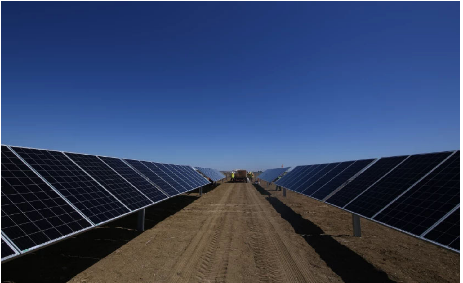
A view of the construction site of Westlands Solar Park on June 24. (Gary Kazanjian / For The Times)
