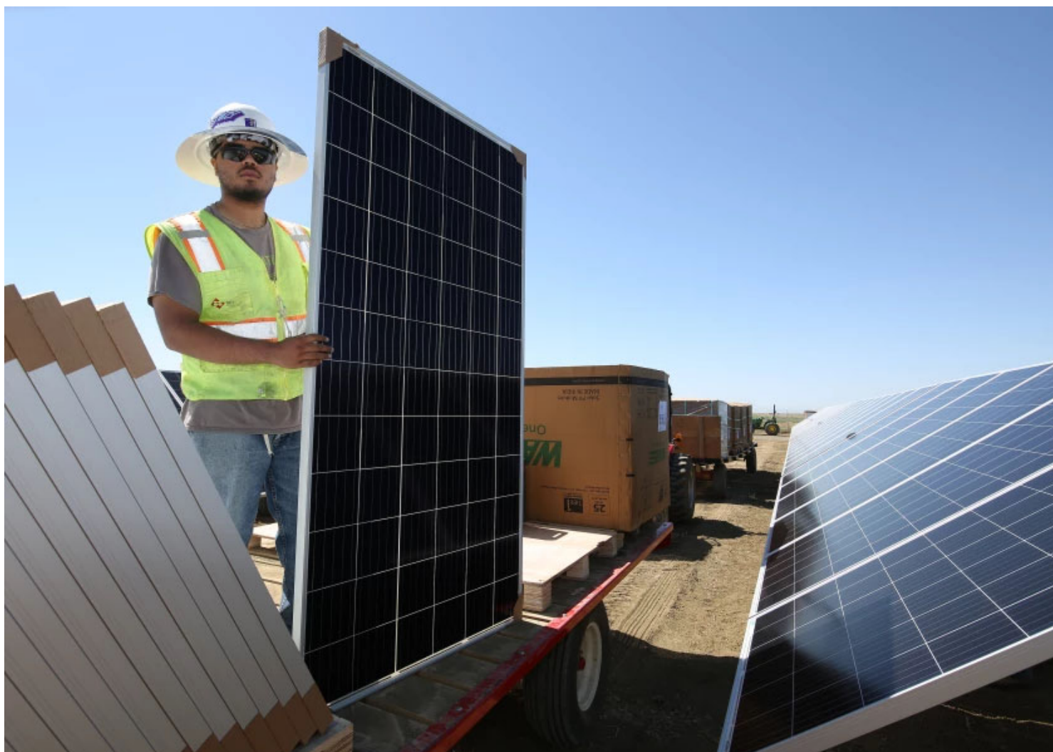
Ricky Figueroa places photovoltaic panels at the construction site of Westlands Solar Park on June 24, 2021. (Gary Kazanjian / For The Times)
