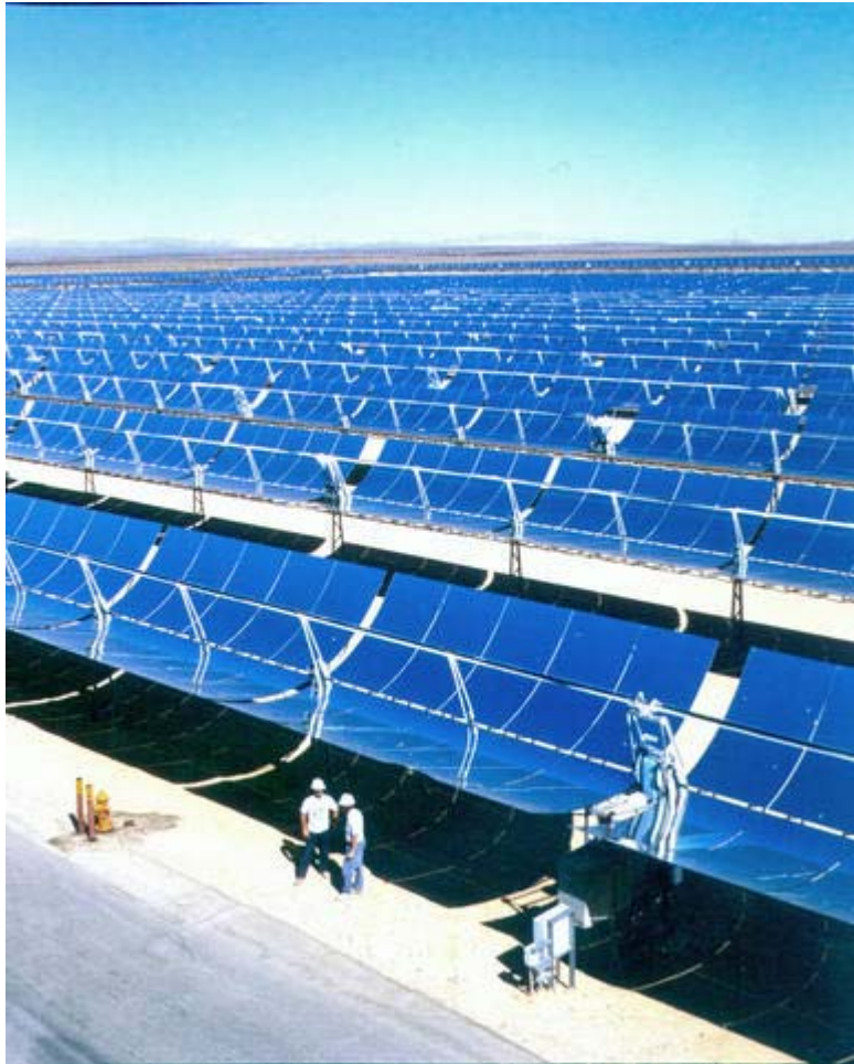
Figure A-2 Kramer Junction Trough Plant (Source: NREL)
