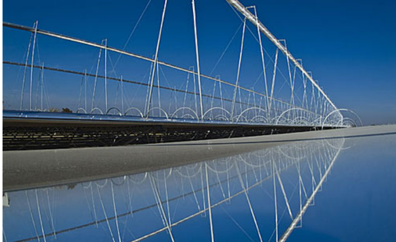
Figure A-5. Compact Linear Fresnel Reflector Power Plant, Kimberlina, California (Source: Ausra, Inc.)
