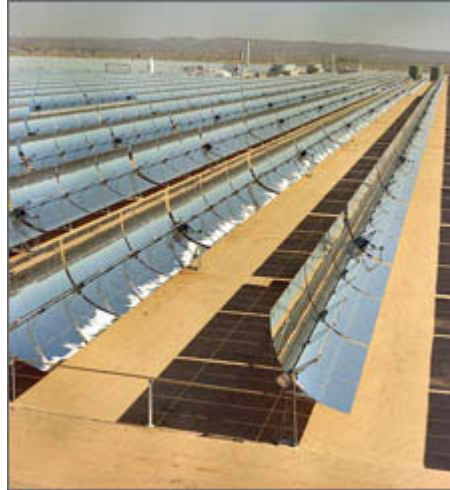
Figure A-2. Parabolic Trough Solar Thermal Power Plant, Kramer Junction, California (Source: National Renewable Energy Laboratory)
