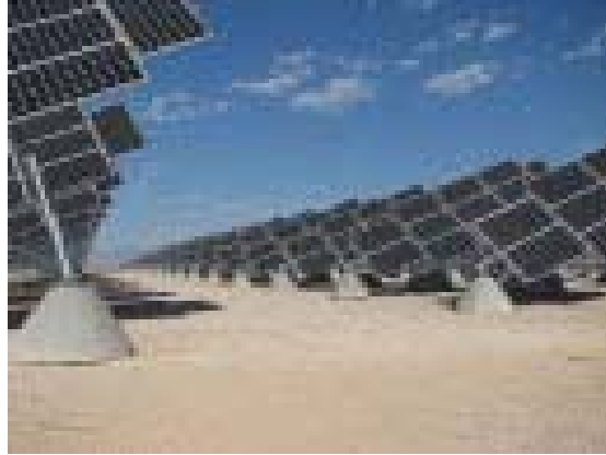
Figure A-6. 15 MW Large-Scale Photovoltaic Power Plant, Nellis Air Force Base, Nevada (Photo: Courtesy of Sunpower Corp.)
