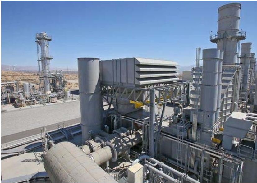
The 800-megawatt Sentinel power plant in Desert Hot Springs, which burns natural gas, is designed to provide power during blackouts and when demand exceeds supply. (Photo: Jay Calderon/The Desert Sun)
