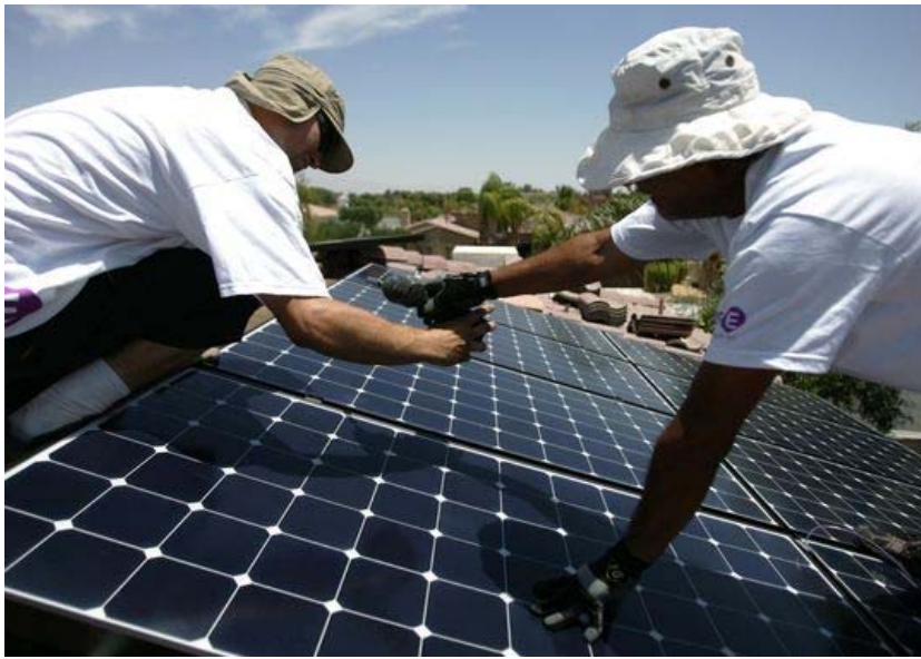
Solar panel installers with Hot Purple Energy (Paul Lemon, right, of Morongo Valley and Phillip Wittwer) bolt on solar panels in a 54 panel home installation job in Rancho Mirage, Wednesday, May 23, 2012. (Richard Lui/The Desert Sun) (Photo: Richard Lui/The Desert Sun)
