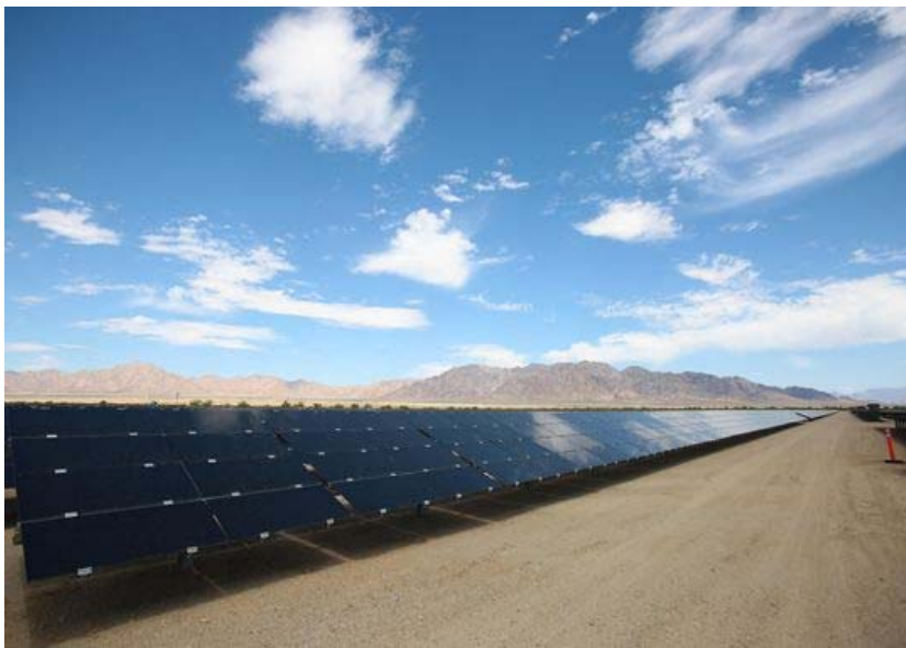
A row of solar panels reflects clouds overhead at the 550-megawatt Desert Sunlight solar farm in Riverside County. It's one of 52 large-scale renewable energy projects on federal land approved by President Barack Obama's administration. (Photo: Crystal Chatham/The Desert Sun)
