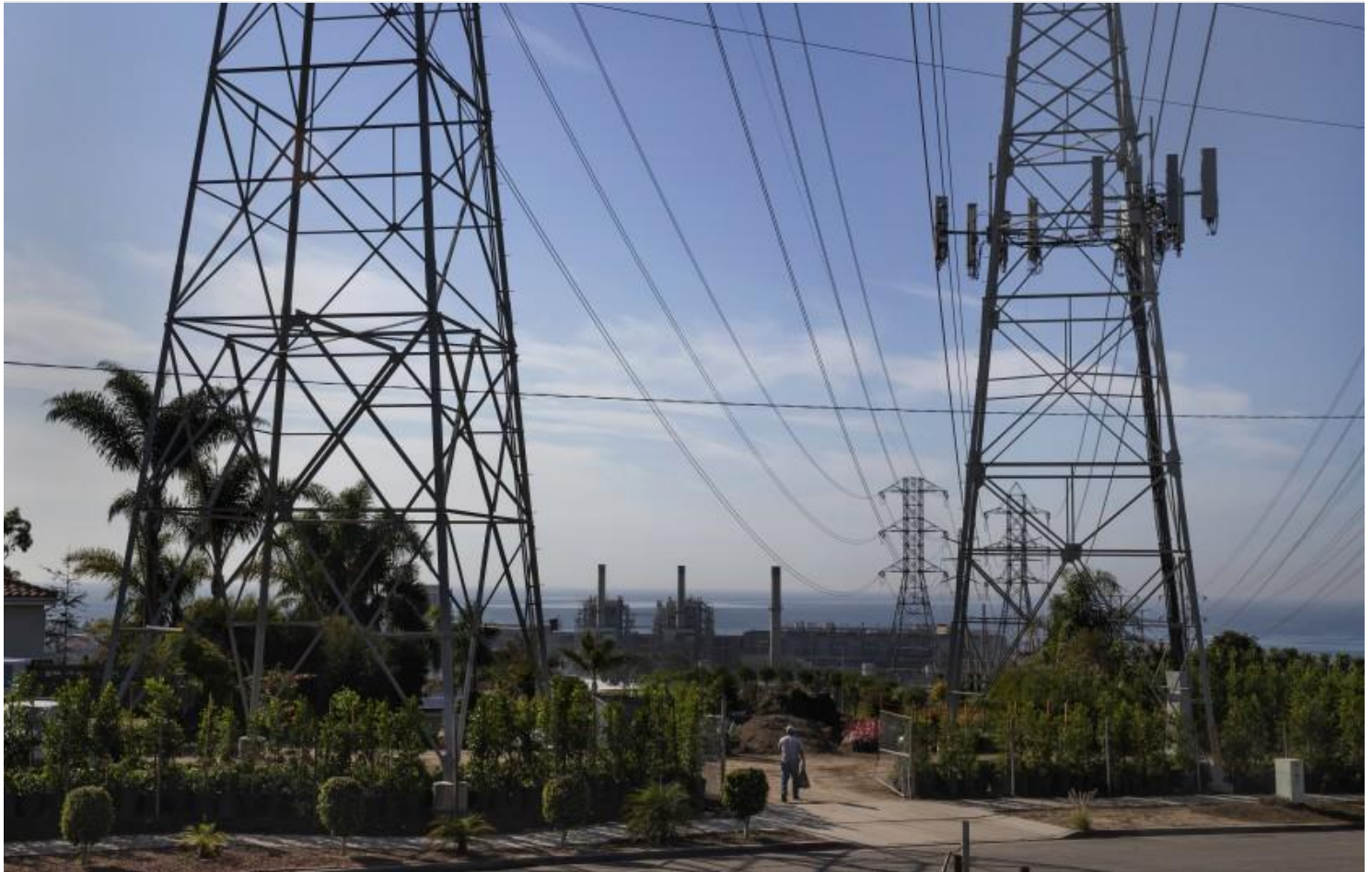
Power lines carry electricity away from the gas-fired power plant in Redondo Beach in 2019. (Mel Melcon / Los Angeles Times)
