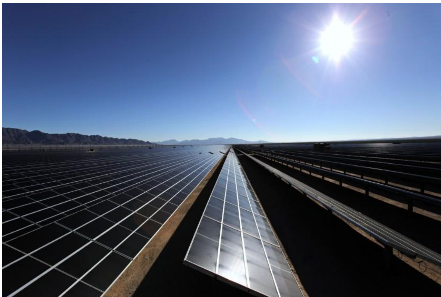
The sun rises over solar panels at the 550-megawatt Desert Sunlight solar farm in Riverside County, California. (Marcus Yam / Los Angeles Times )
